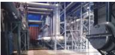
EHV Gas Insulated Substation (GIS)
